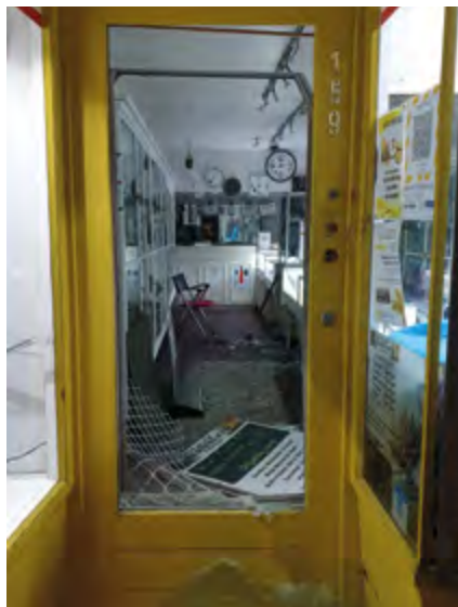
DM's front door opens to damage within.
